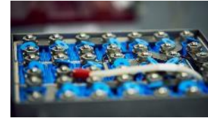
Batteries and Chargers
